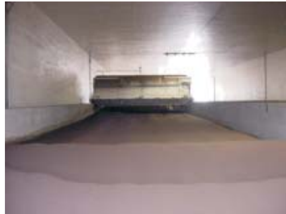
Compost turners lift and mix the material and move the composting material along the channel. Photo Courtesy: Transform Compost Systems Ltd.
