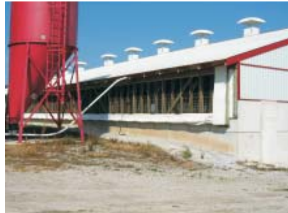
Insulated sidewall panels and roof chimney vents. Photo Courtesy: Agviro Inc.
