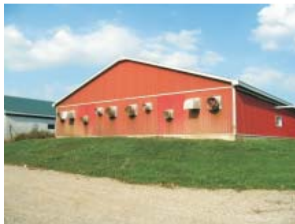
Mechanical fans exhausting from building. Photo Courtesy: Agviro Inc.
