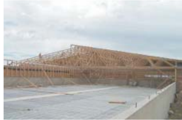
Typical construction involves concrete foundation elements with wood wall and roof. Photo Courtesy: Miles Jorgenson
