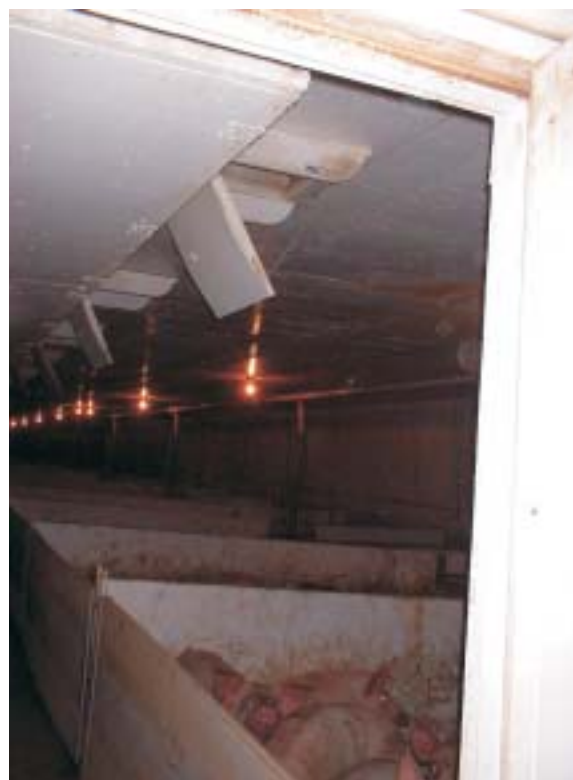
Air inlet directing air to pens. Photo Courtesy: Agviro Inc.
