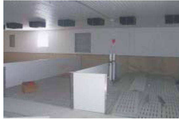
PVC penning and wall liners reduce cleaning time and water use.
